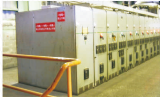
興達發電廠 Shin Da Power Company
