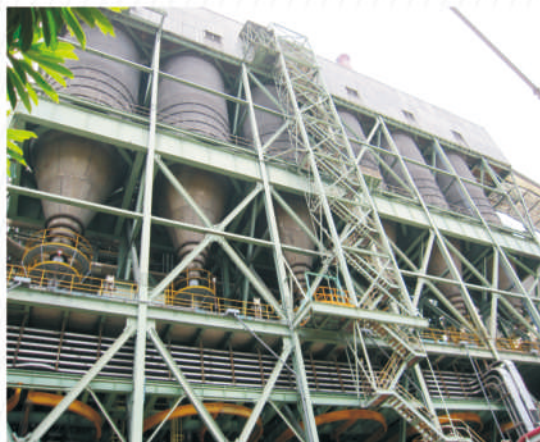
興達電廠 Shin Da Power Company
