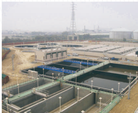
路科汙水處理廠 Southern Taiwan Science Park
