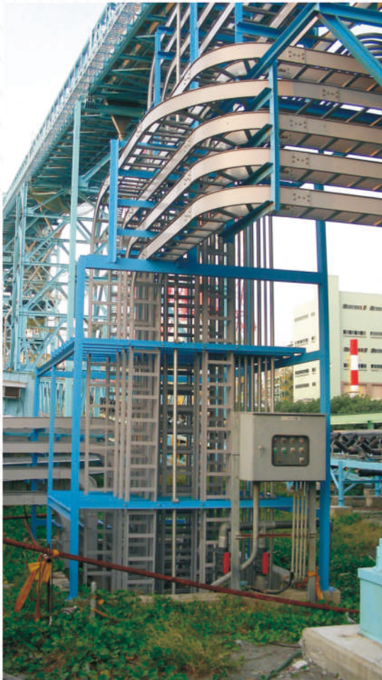
興達發電廠 Shin Da Power Company
