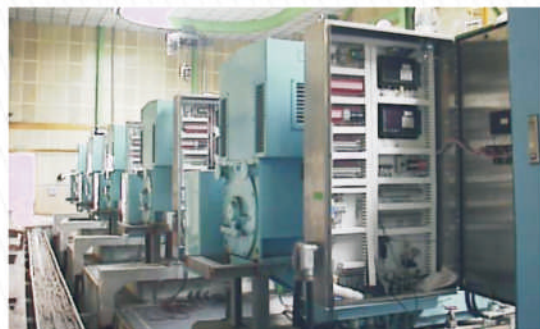
興達發電廠 Shin Da Power Company
